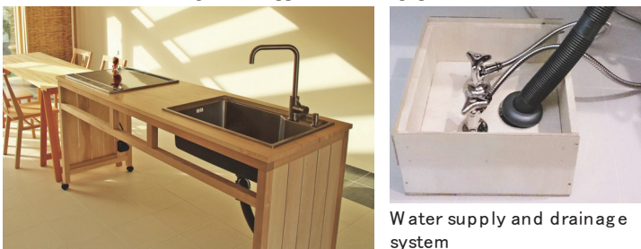
Figure 14 Inside of the kitchen and living room (left) and water supply and drain pipes (right).
